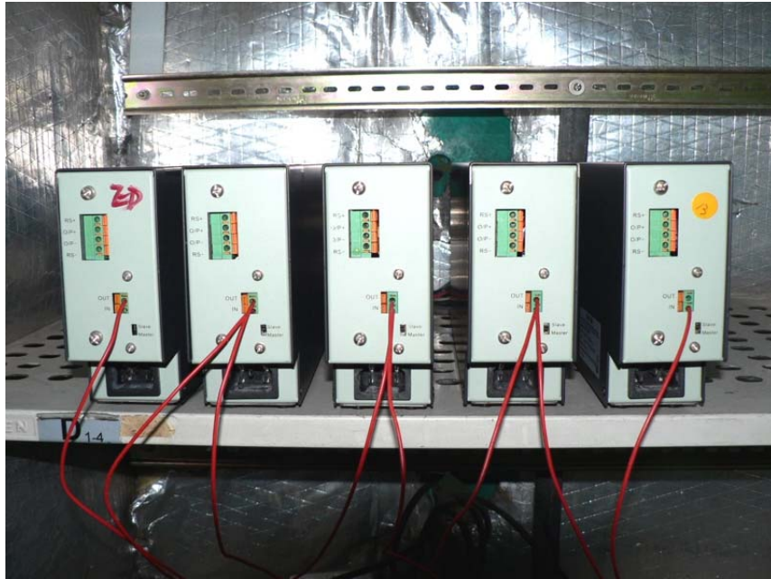
Figure 3 Setting of Master and Slave connections at the rear panels of 5 units of SSP-7080 modular power supplies
